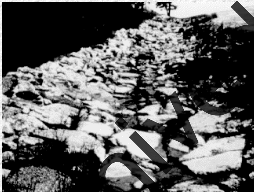
Figure 8. Broken Concrete Riprap
